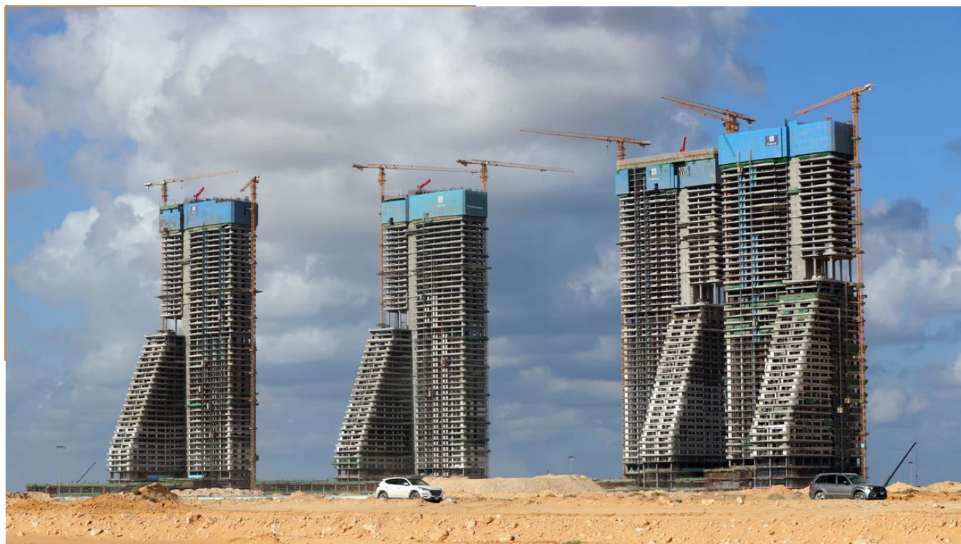
The construction site of the Alamein Downtown Towers Project in New Alamein City, Egypt [Xinhua News].
