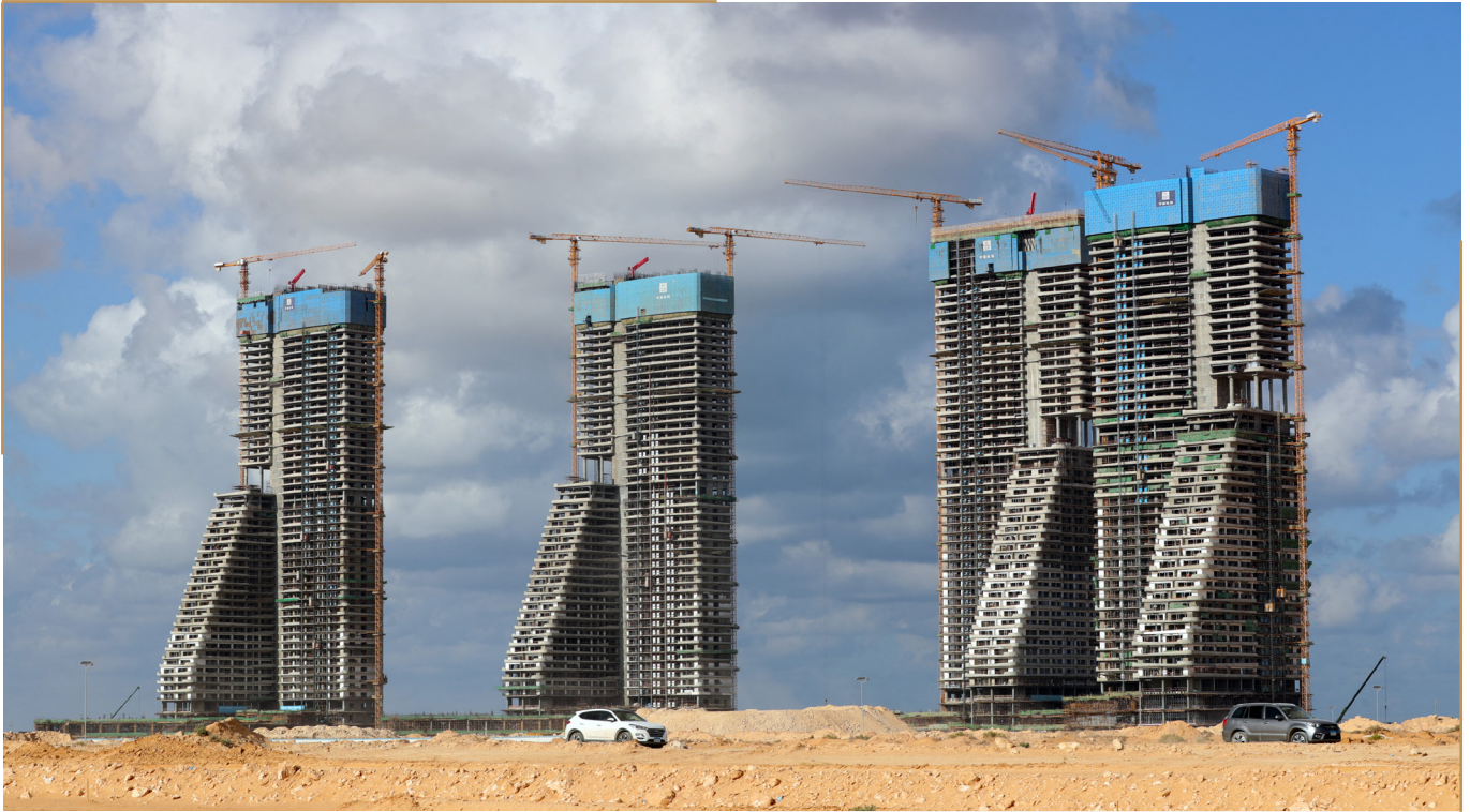
The construction site of the Alamein Downtown Towers Project in New Alamein City, Egypt [Photo by Sui Xiankai / XINHUA / Xinhua via AFP].
